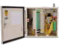
CE Splitter Cabinet
