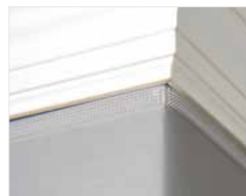
Clear Track Quad Fiber Pathway Installed Around Exterior Corner
